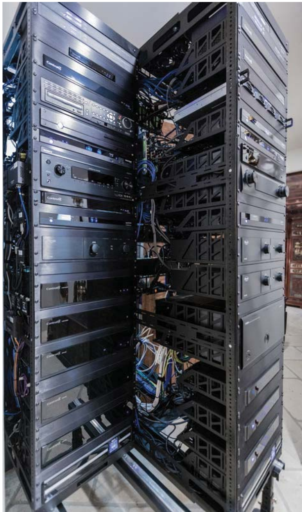
An HC-800 controller and two HC-250 controllers power the system from a climate-controlled rack room, automating everything from ice machines to aquariums.
